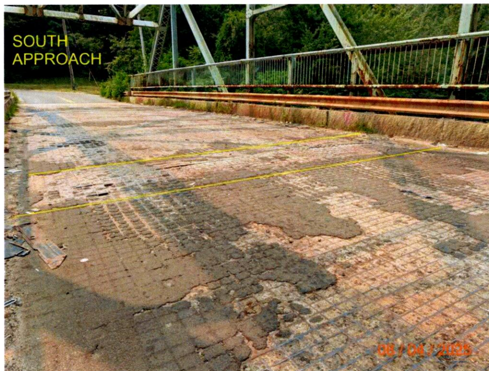
Photo 4: Steel Grid Deck is buckled above Floorbeam FB3.
