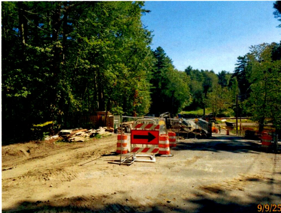
Photo 5: West At-Bridge signage, typical condition. Currently under active construction.
