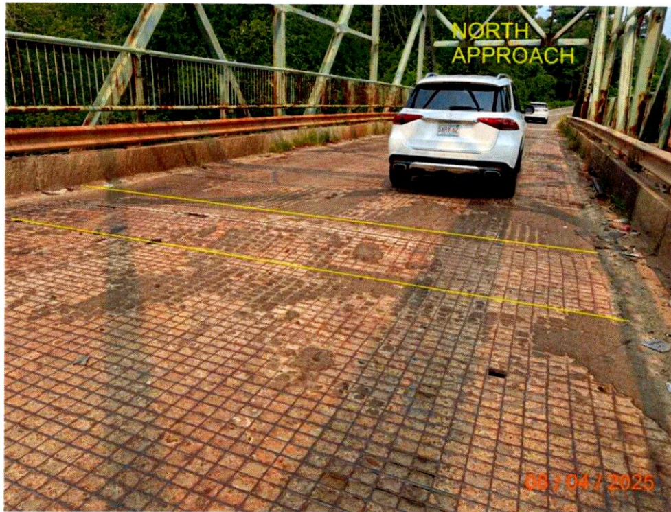
Photo 5: Steel Grid Deck is buckled above Floorbeam FB3.
