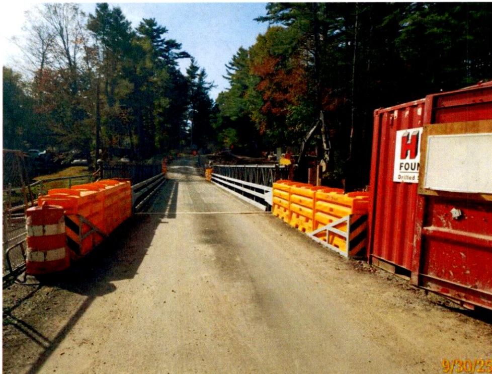
Photo 18: Transitions consist of a 3 barrel Sentry Longitudinal Energy Dissipater (SLED) system.
