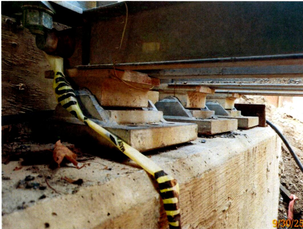
Photo 15: East Bearings (expansion) do not have anchor bolts. Each of the 3 web panels rest on an individual bearing.
