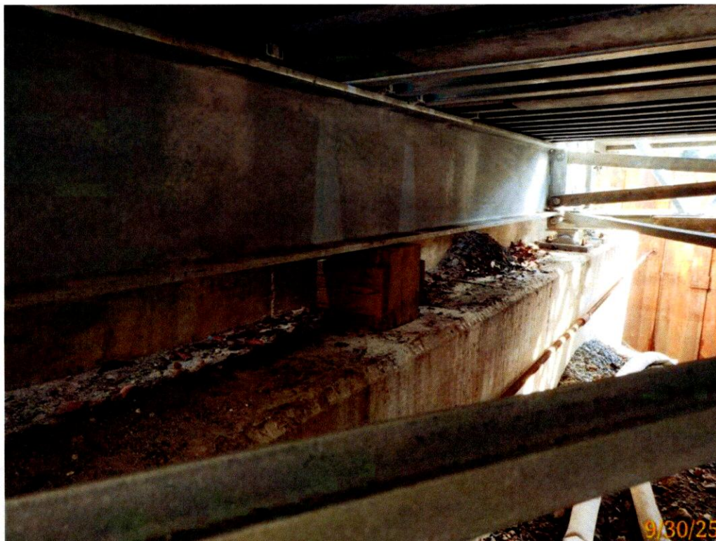
Photo 16: East Bridge Seat has minor sand accumulation. Both seats have timber blocks that act as bolsters per the plans.
