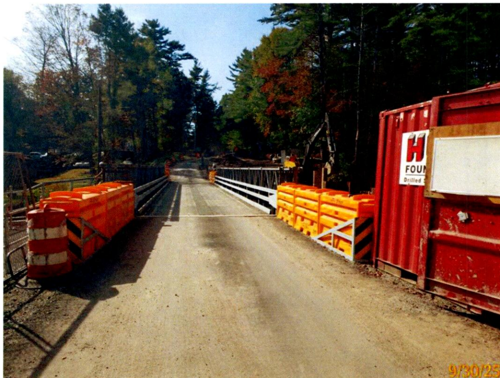
Photo 18: Transitions consist of a 3 barrel Sentry Longitudinal Energy Dissipater (SLED) system.
