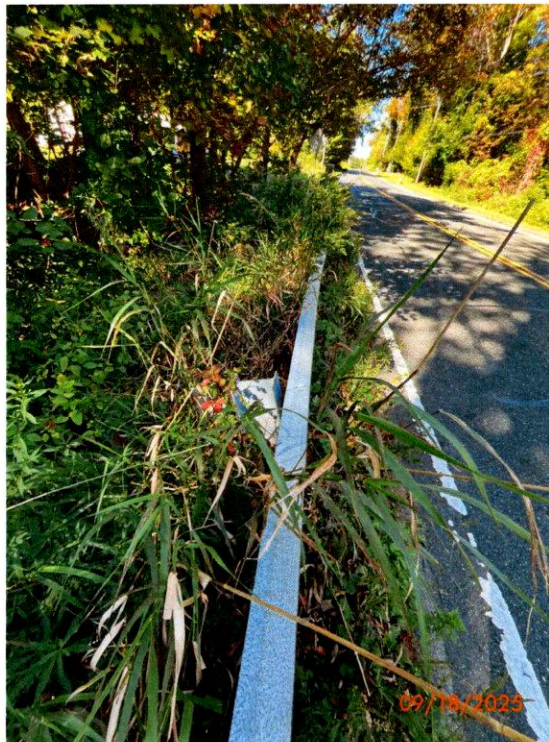
Photo 10: Northwest Approach guardrail has moderate collision damage. Guardrail is leaning to the west.
