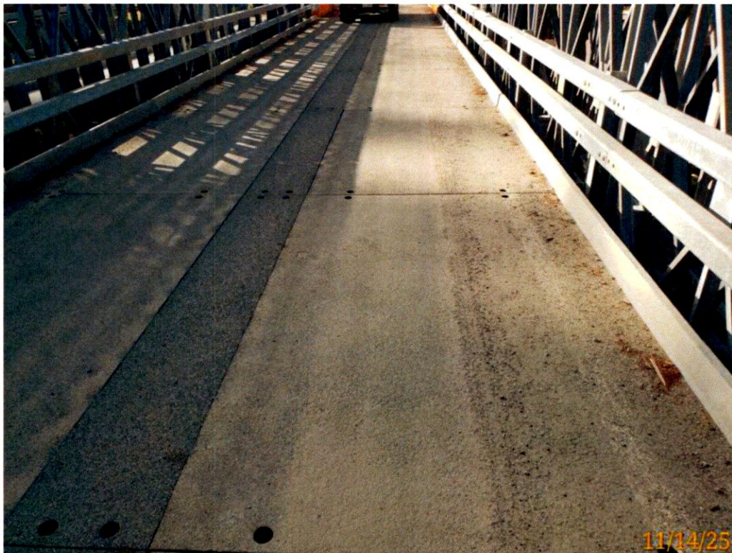
Photo 4: Wearing Surface has minor sand and debris.
