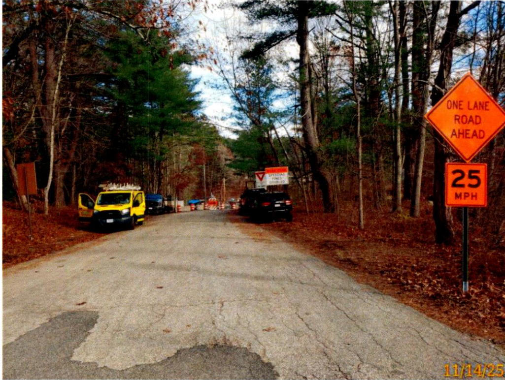
Photo 3: West Advanced Signage, typical condition.
