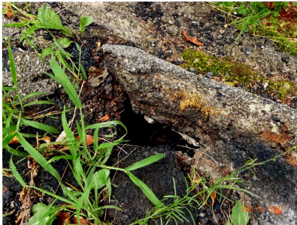
Photo 4: Southwest Approach, along curb has void towards west wingwall and towards roadway.
