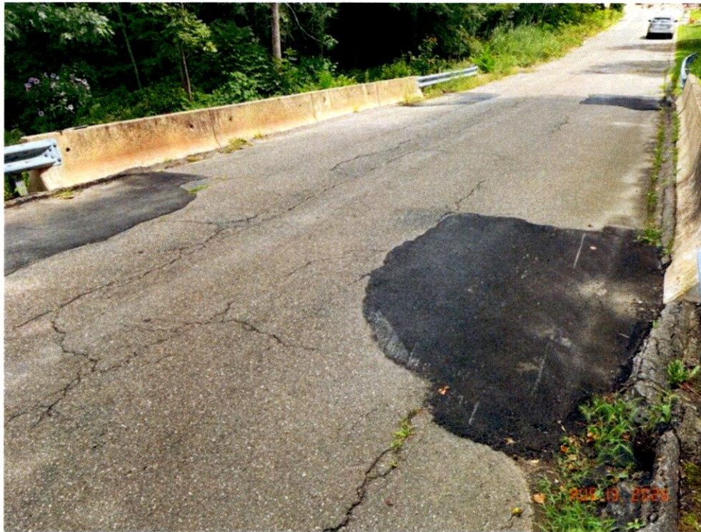
Photo 1: Wearing Surface at all four corners, adjacent to the approaches, has patching & settlement, up to 3" deep.
