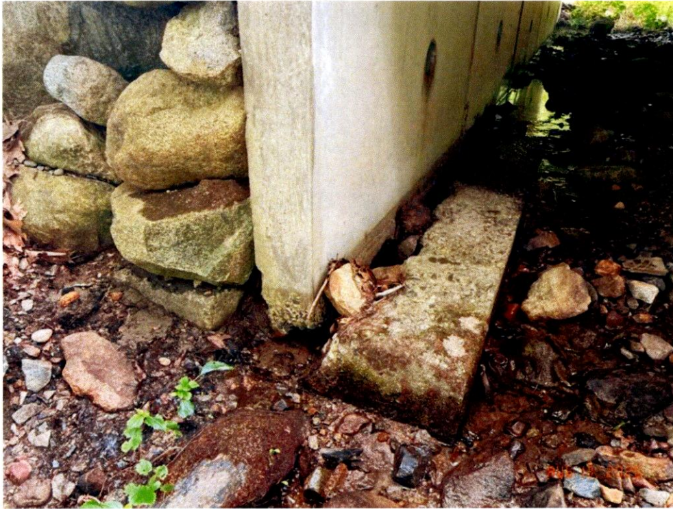
Photo 7: Rigid Frame, west side, is undermined with scaling.
