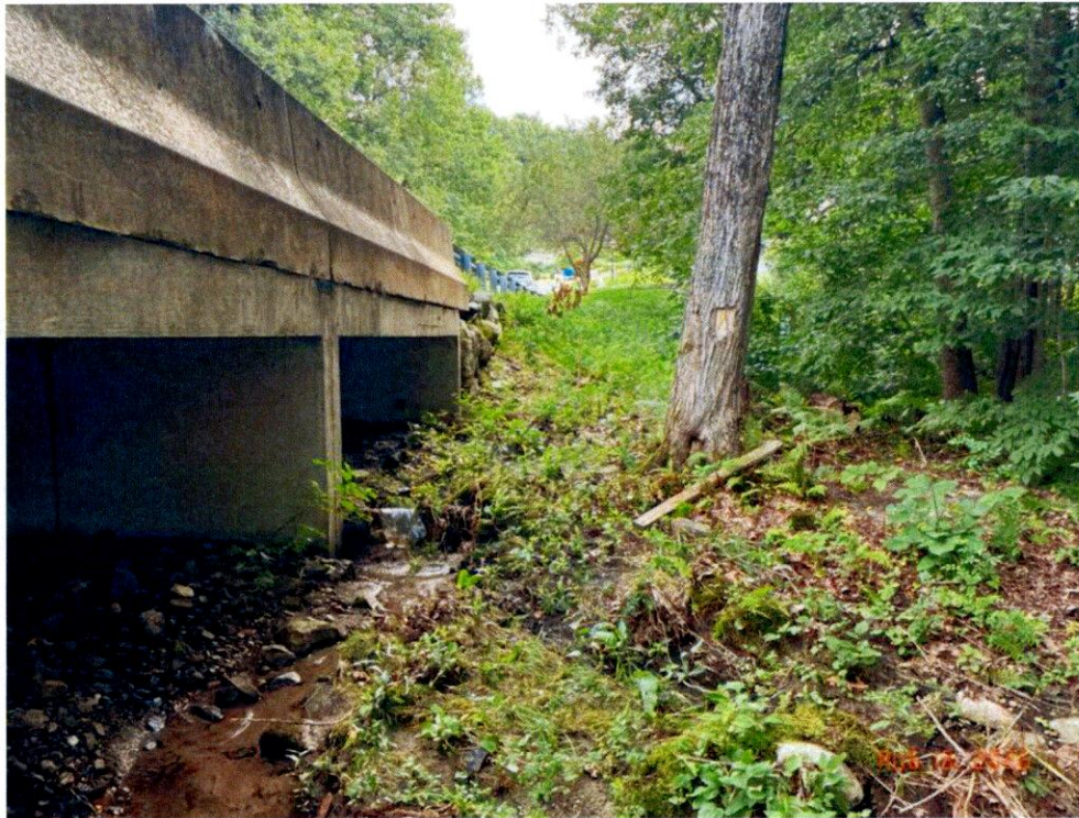
Photo 13: Both elevations have minor to moderate vegetation growth.
