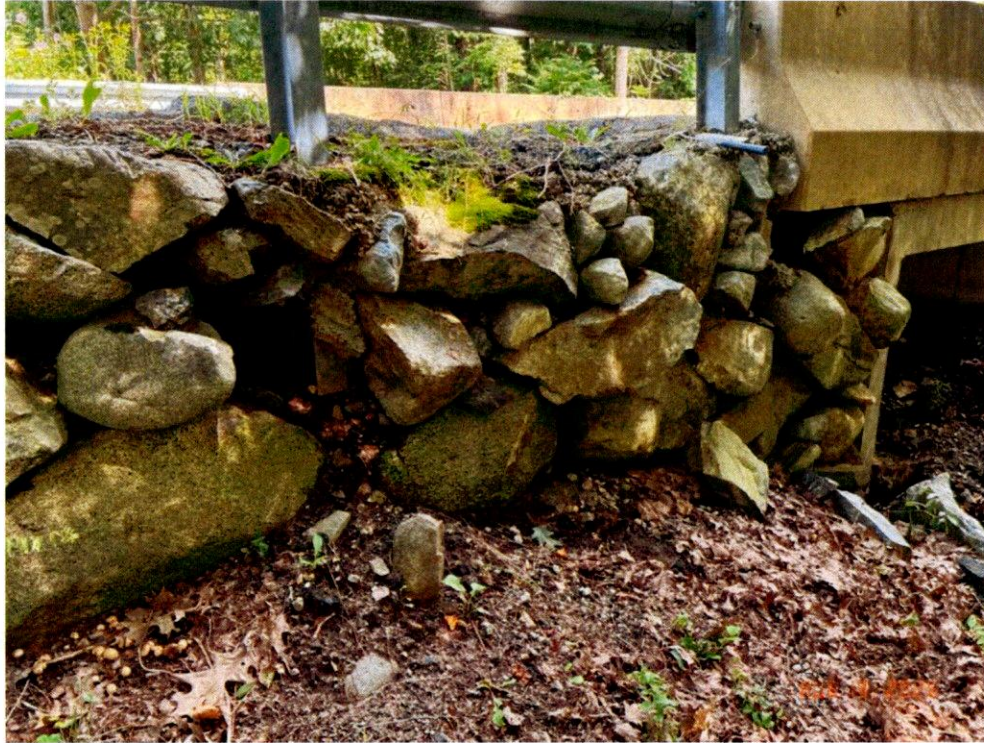
Photo 11: Guardrail Post, 2nd from Bridge, underside has void with guardrail post floating.
