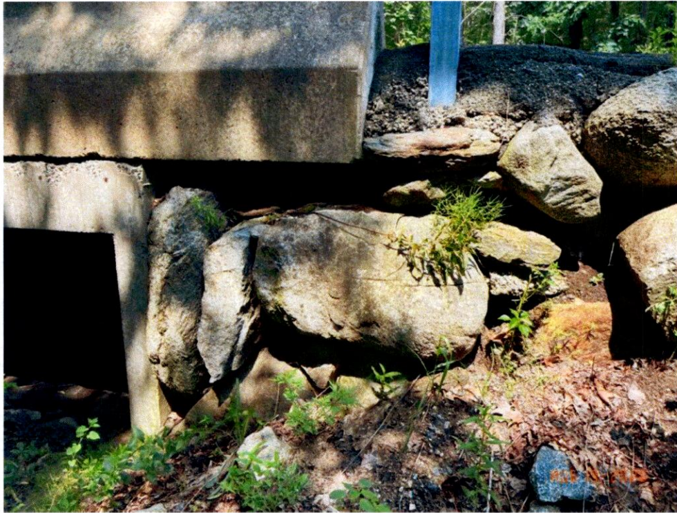
Photo 9: Southeast Wingwall has settlement with missing stones. Frame headwall has chipping.
