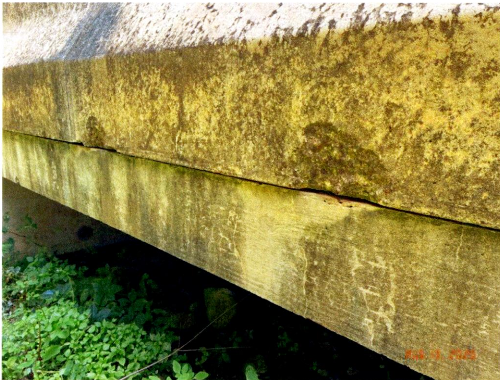
Photo 2: Parapets have small spalls along the outer edges of the barriers.
