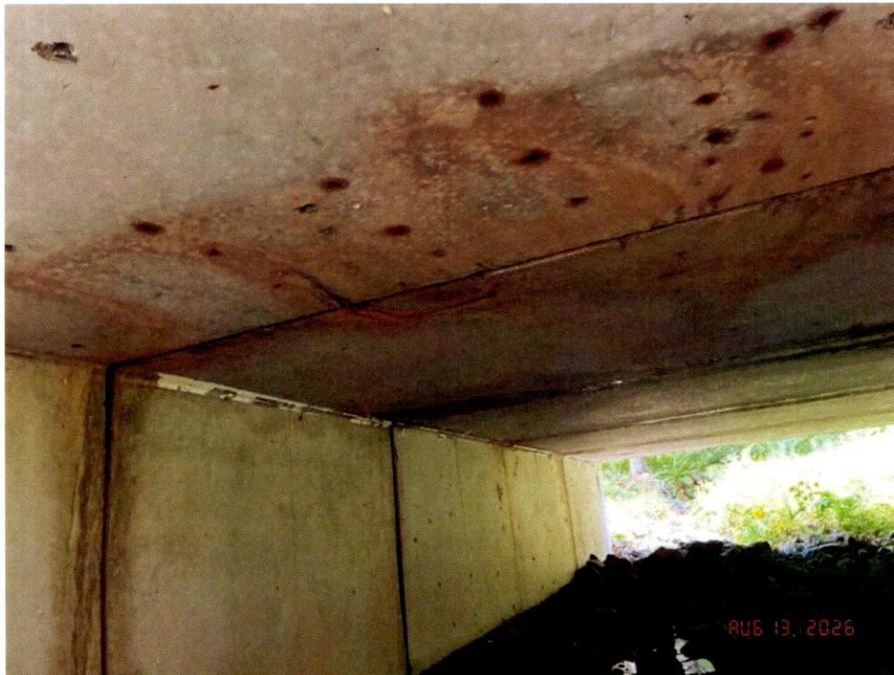
Photo 8: Frame 2, underside has minor water & rust stains between the joints.
