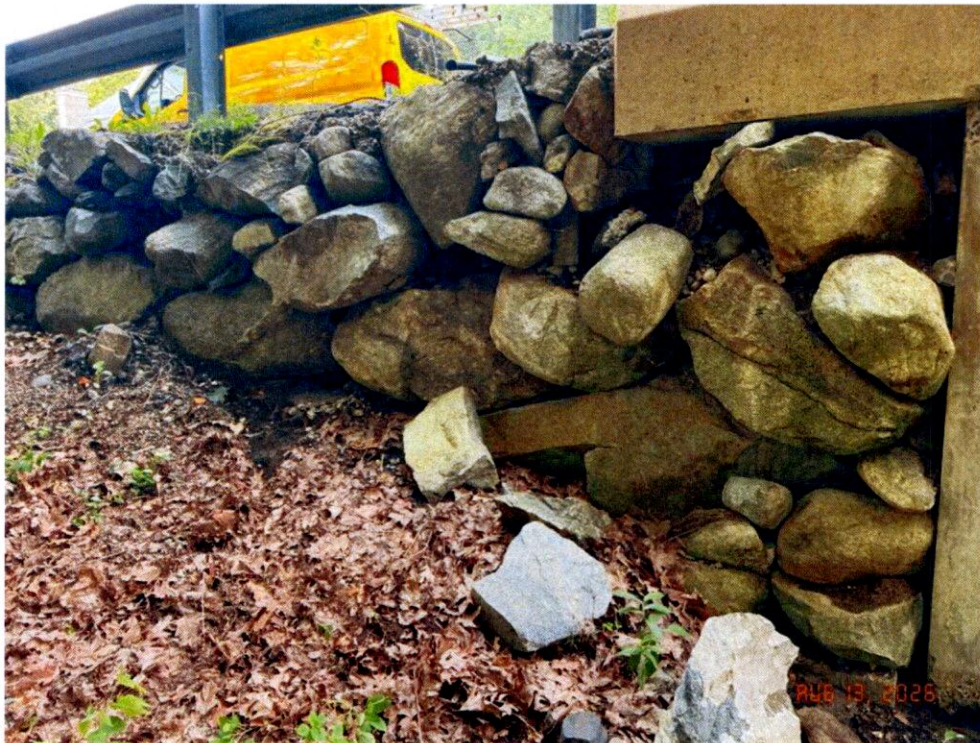
Photo 10: Southwest Wingwall has stones that have fallen out and are shifting.
