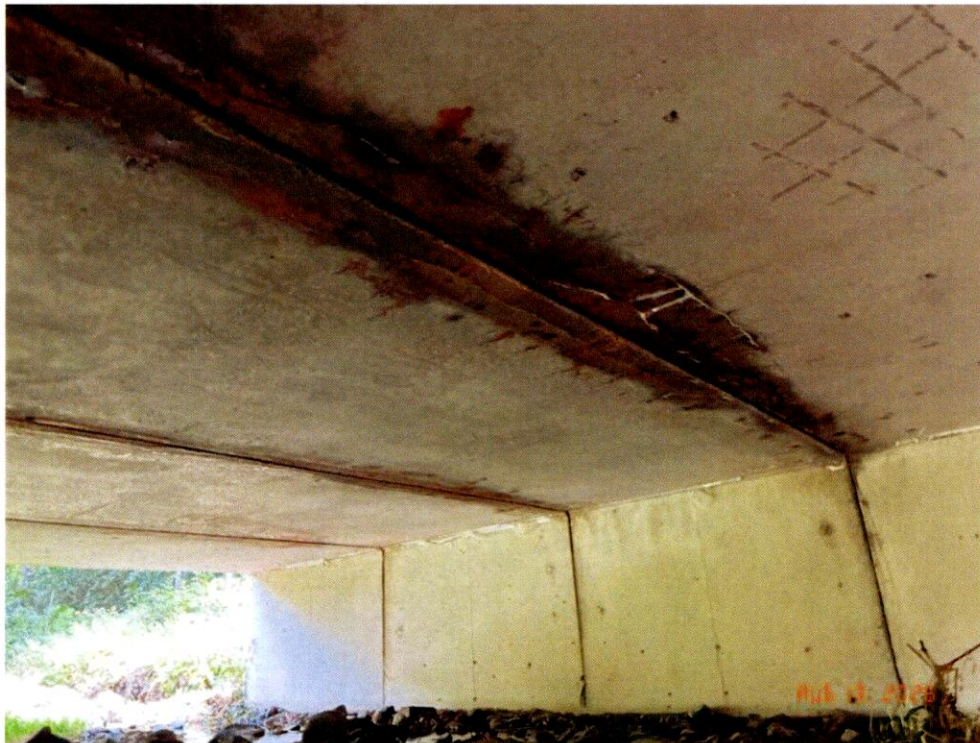
Photo 6: Frame 1, underside between Sections 2 & 3 has water/rust stains and cracking along the joint.
