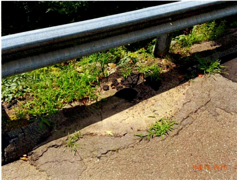
Photo 5: West Deck End, south side, has erosion & settlement with cracking.
