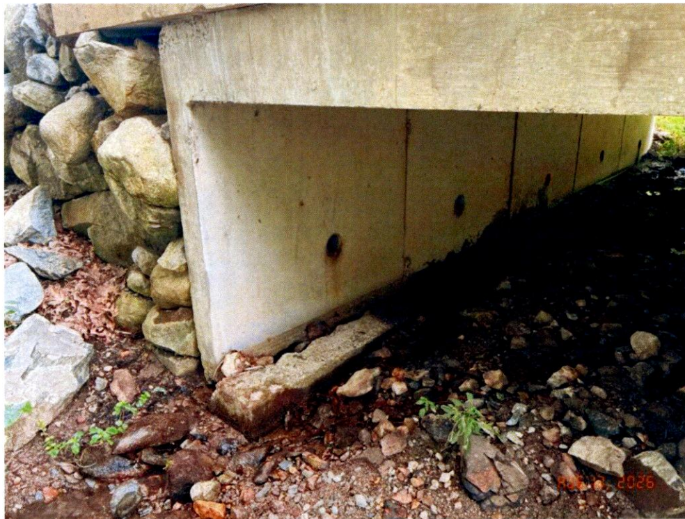
Photo 12: Frame 1, southwest corner, footing is exposed for a length of 17'.
