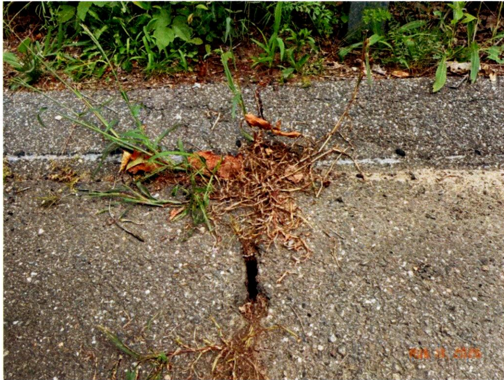
Photo 3: West Approach, North side, has transverse cracking full width with void.
