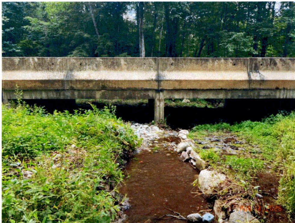
Photo 14: Upstream Channel has aggradation reducing openings by up to 50%.
