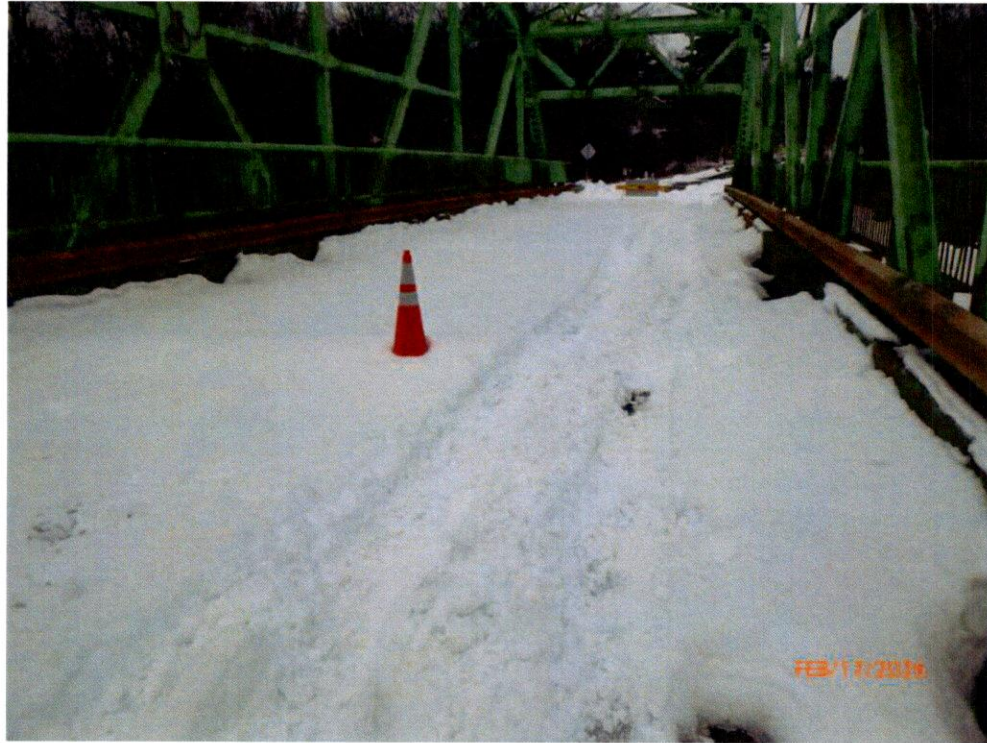
Photo 1: At Panel Point 3, there is a heave in the deck which is buried in snow.
