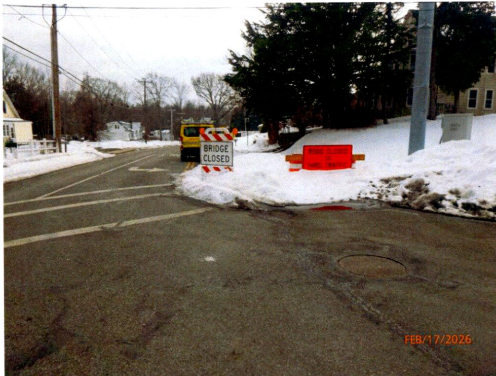
Photo 4: North Advance at Intersection (West Street & West Avenue/Russell Street): 2 barrels, 1 ("Road Closed to Thru Traffic") & 1 Hazard Barrier w/ ("Bridge Closed") sign attached.
