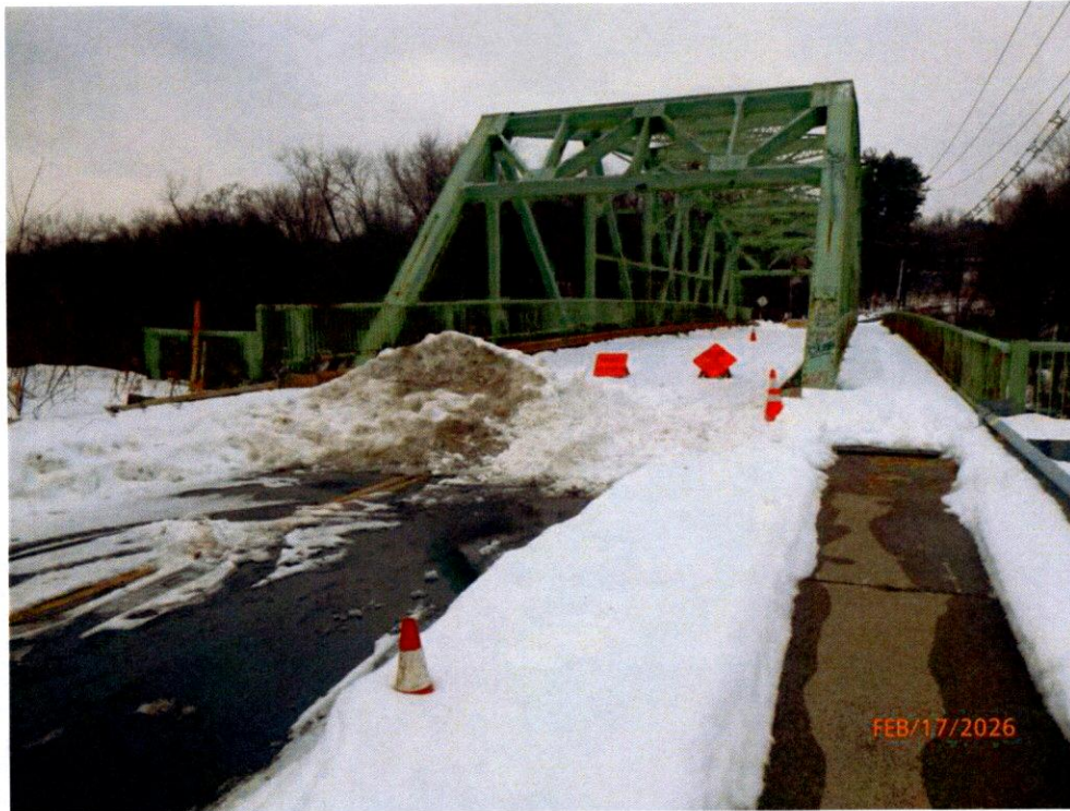
Photo 3: South Bridge Approach: Barriers unknown due to large snow bank. Signs ("Bridge Closed") & ("Warning Bump on Bridge Ahead") are beyond the snow bank.
