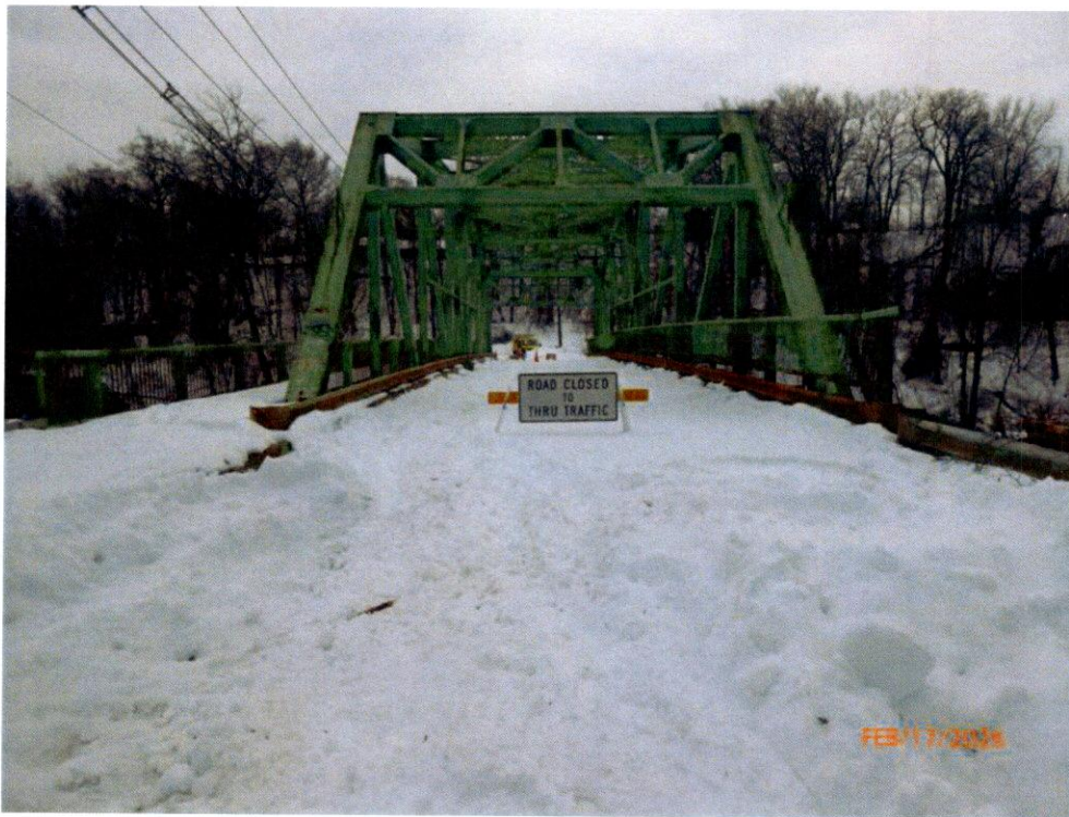
Photo 6: North Bridge Approach: 1 ("Road Closed to Thru Traffic") sign.
