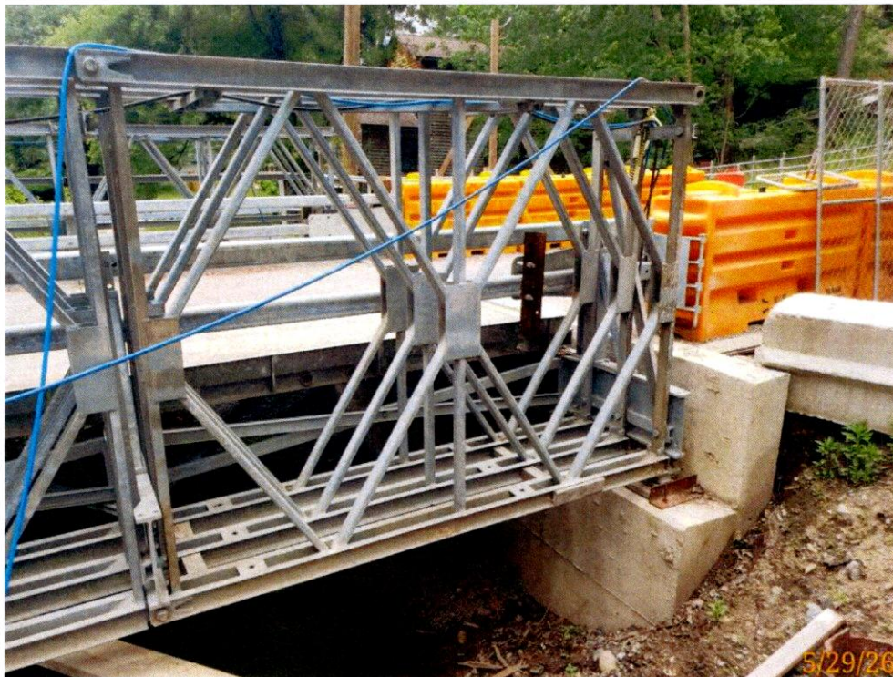
Photo 6: East Bridge Seat has minor sand accumulation. Web members have minor corrosion.
