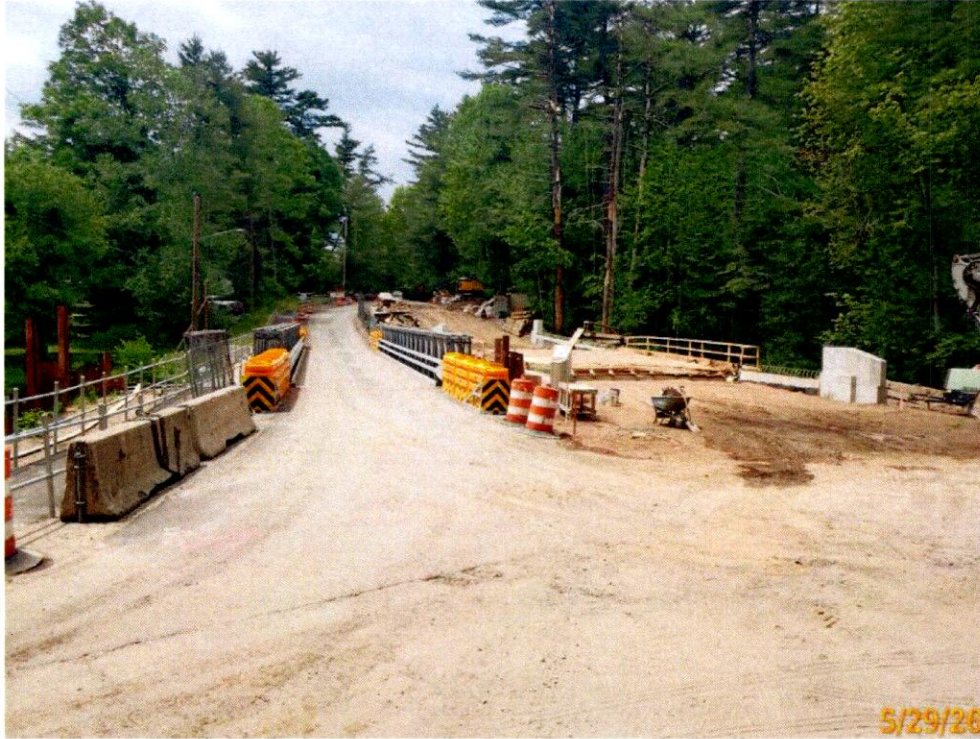
Photo 1: Pedestrian and Highway traffic is directed onto and ACROW panel. The construction site has barriers removed during active construction.
