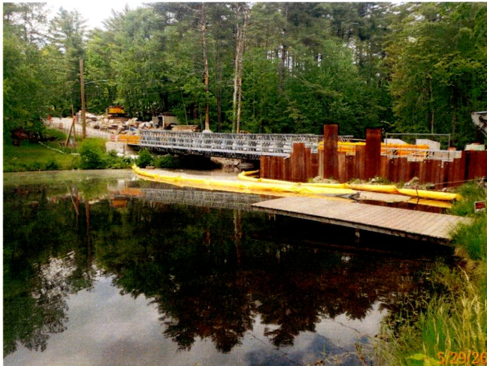
Photo 4: Water level has been raised to summer level, underside of structure is mostly inaccessible.
